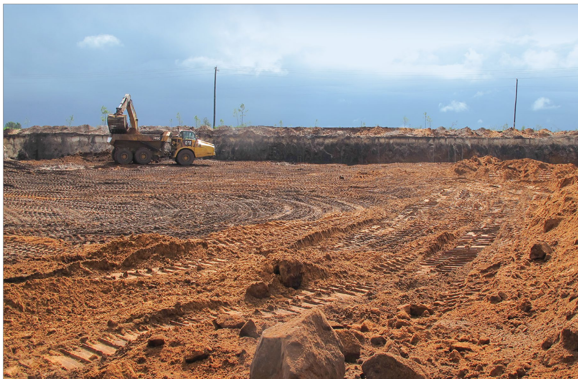
Figure 35: Dry mining at Southern Ionics Minerals' Mission South mine in August 2017. Photo: BGR.
